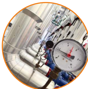
Heat exchange unit
